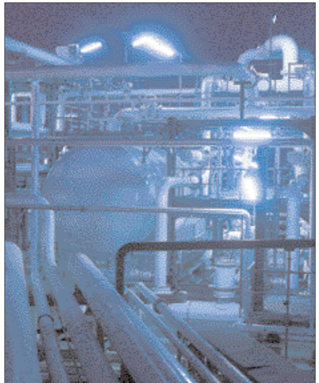
Varanus Island Gas Plant
