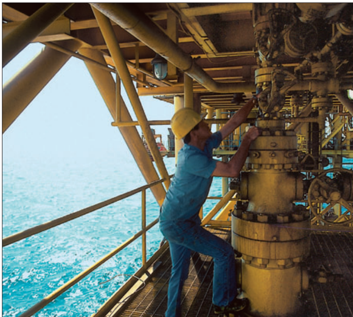
More than 3,000 production platforms now produce crude oil and natural gas in the Gulf of Mexico. Compact, self-contained structures, they rise about 35 feet above water and contain everything needed for offshore operations, including helipad and crew’s quarters.
