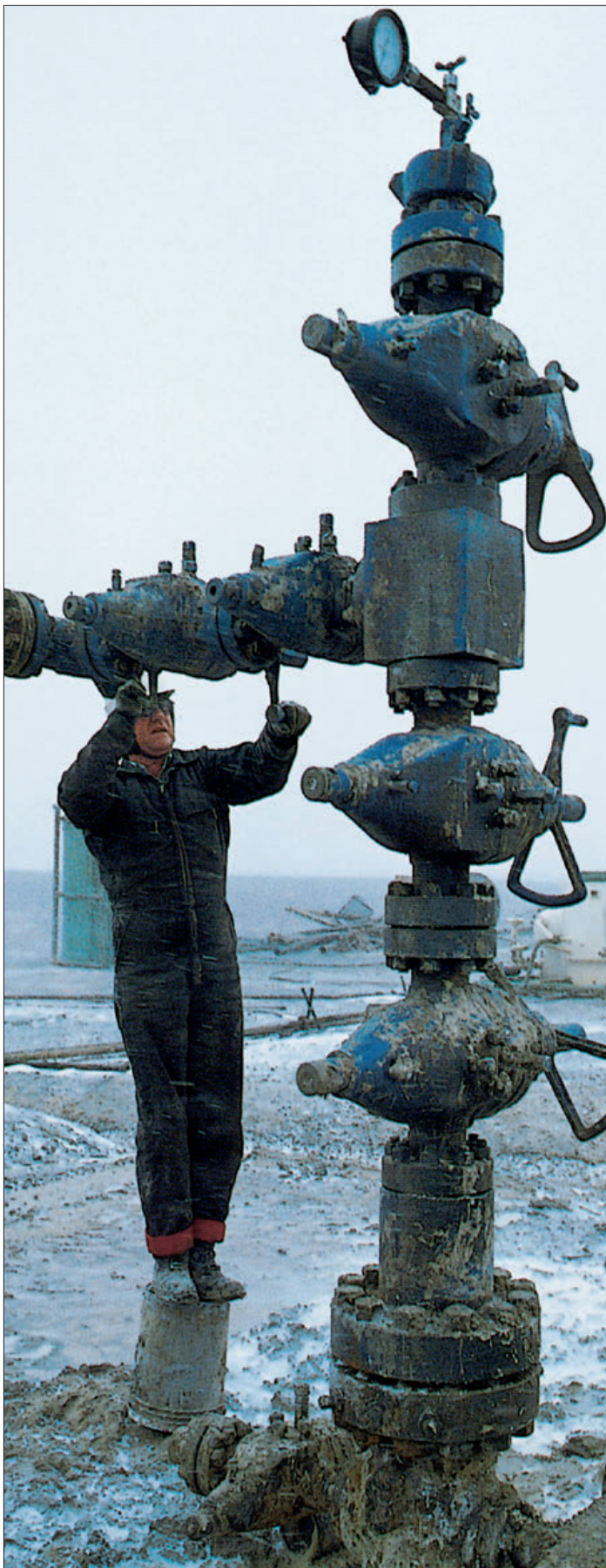
The raw, wet winter winds in the Texas Panhandle didn't delay pipeline hookup of this Anadarko Basin gas discovery.
