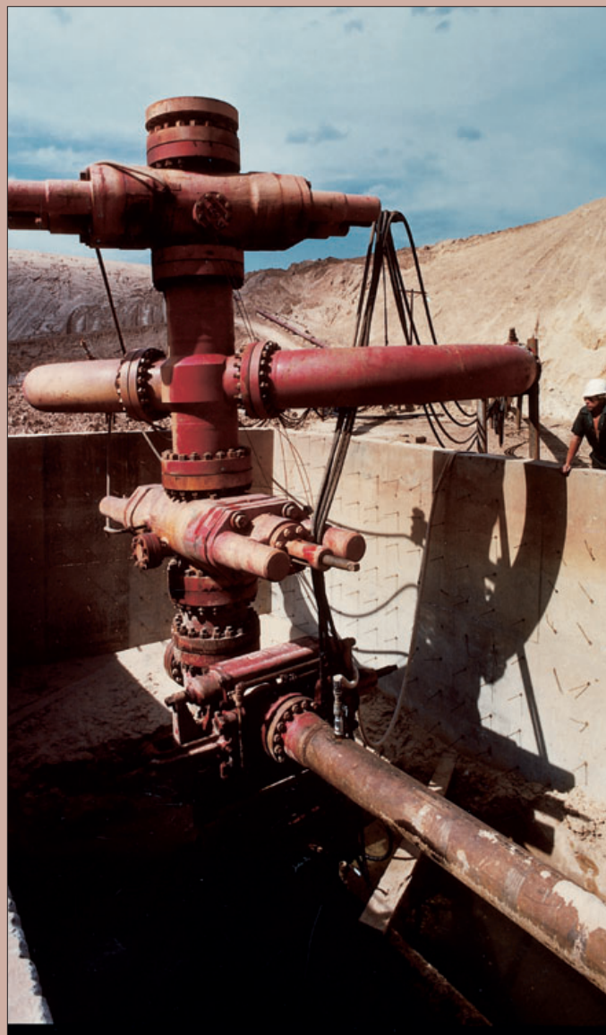
Temporary production facilities at Apache’s Key # 1-11 in Wheeler County, Texas, included this structure on the wellhead and a series of mechanical scrubbers and compressors. The well produced over 30 million cubic feet of gas per day as a controlled blowout for eight months until it was killed below ground through a relief well in early 1983. A replacement well was completed several months later.
